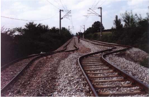
Figure 5: 230 cm horizontal deformation near railway station Tepetarla in the region between Sapanca Lake and Izmit Gulf (Source: Esen Arpat, Kandilli observatory).
