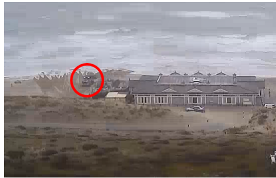
(b) A bulldozer is present and working in the area of deformation.
