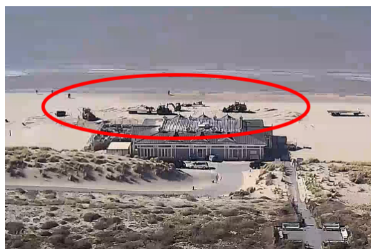
(b) A lot of heavy equipment is present and working in the area of deformation.
